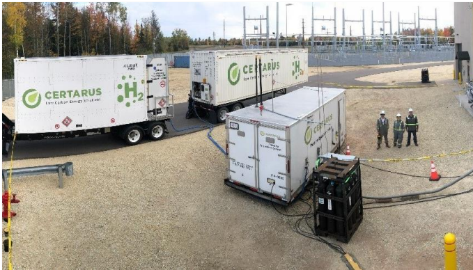
WEC: Supplied H2 for the world's largest H2 test on a grid-connected reciprocating nat gas engine at MI power plant (18% H2 in 18MW Engine – Largest H2 flow to grid connected engine). Revenue = $330k
