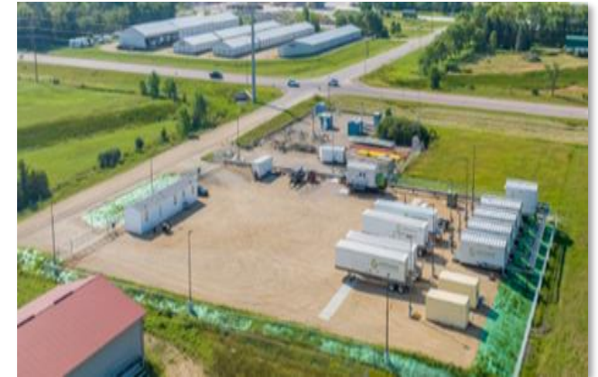
Permanent RNG Injection Station – Fixed pressure reduction and pipeline injection compressors injecting agricultural RNG into pipeline via Certarus injection facility
