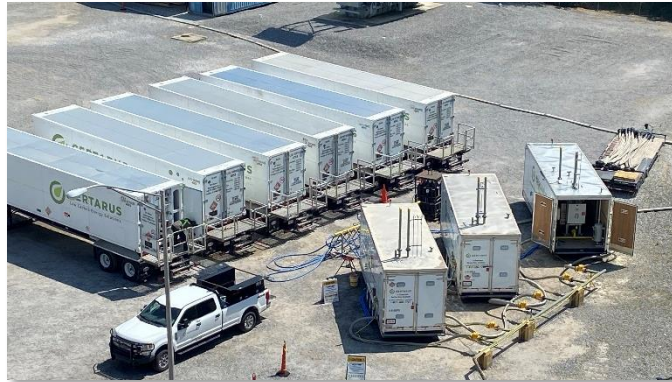
Siemens: Provided on-site H2 delivery to support gas turbine fuel blending test at Constellation Power facility; 39% H2 in 265MW Turbine – Largest H2 flow to a gas turbine (at time of project). Revenue = $1.25MM
