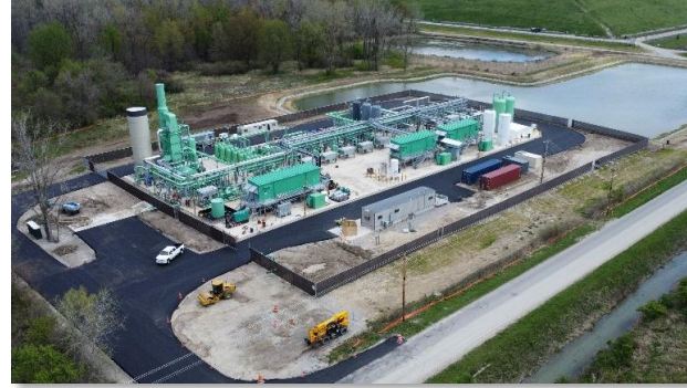
Archaea Republic Services JV – Indiana Landfill: Project recently came online and represents the first trucked project in the Lightning portfolio. Site has been averaging 3-4 loads/day
